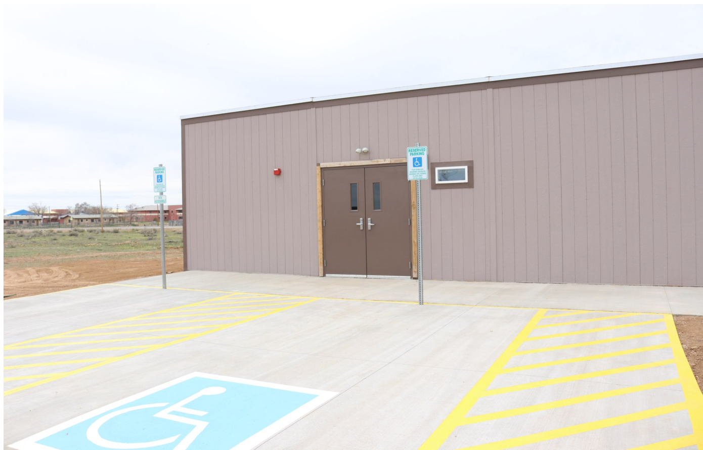
This will be the new Dził Yijiin Judicial District facility in Pinon, Arizona.
